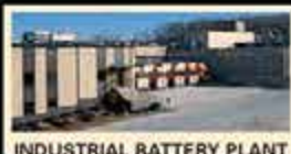
INDUSTRIAL BATTERY PLANT
